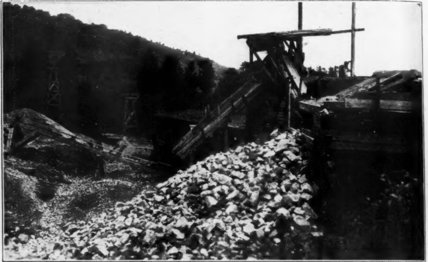
View of Screening Plant—At Right Is Grizzly—Belt Conveyor Under Grizzly Elevates the Sand
